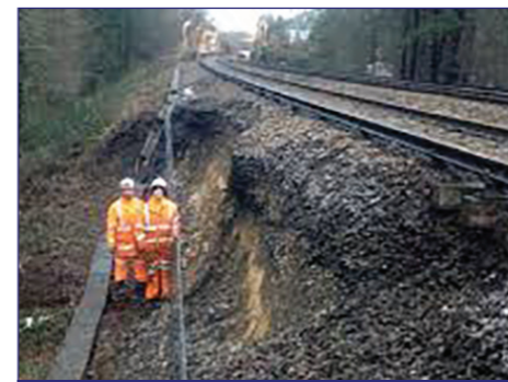
The Nightmare of Collapsed Embankments
